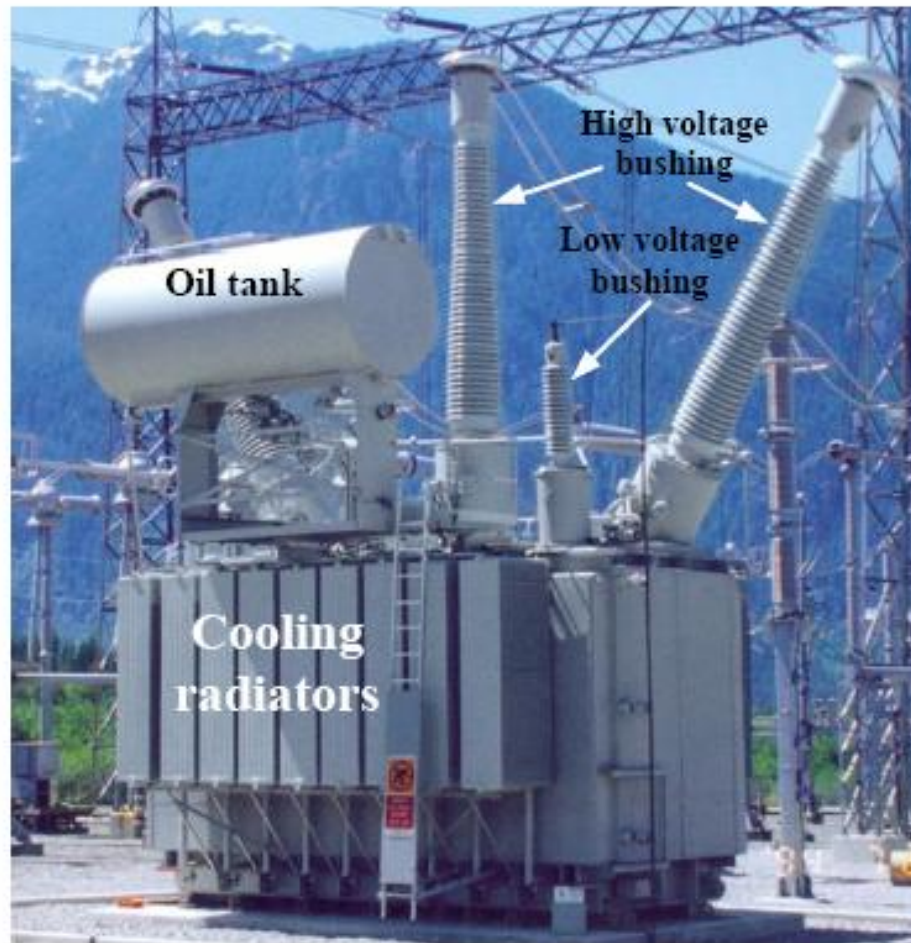
Figure 5.9 Large Oil cooled high voltage transformer
